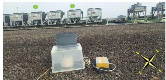
Fig. 11. One of the measurement points for the south side of the reactor building (point FS9). In the northern part of the reactor building, there is an air ventilation chiller system that operates continuously throughout a day to ensure the air quality in the reactor building is consistently maintained. The green solid circle above the ventilation system chiller shows the chiller that was operating at the time the recording was taken.
